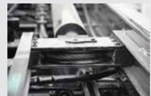
5/8" Cable & 8" Cable sheaves w/ UHMW wear guides
